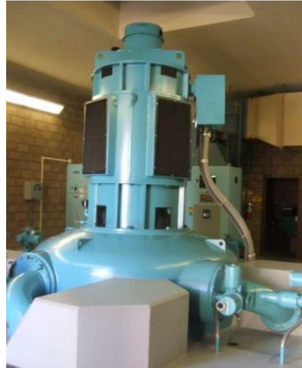
Figure 9-3. San Dimas Hydroelectric Plant Turbine and Generator.
