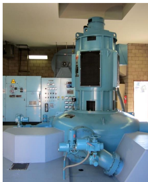
Figure 1.2: San Gabriel District's Hydro Electric Generator at San Dimas Wash
